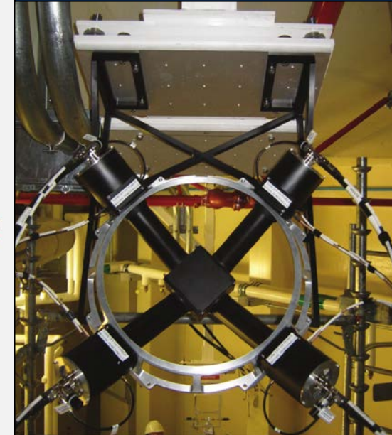
Photo of installed detector
